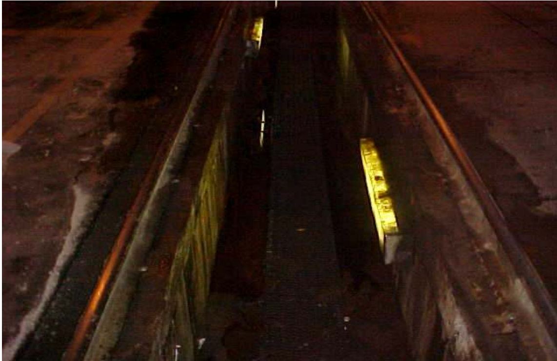
View South - Service Trench collected some of the released diesel on the north end of Service Track 1.
