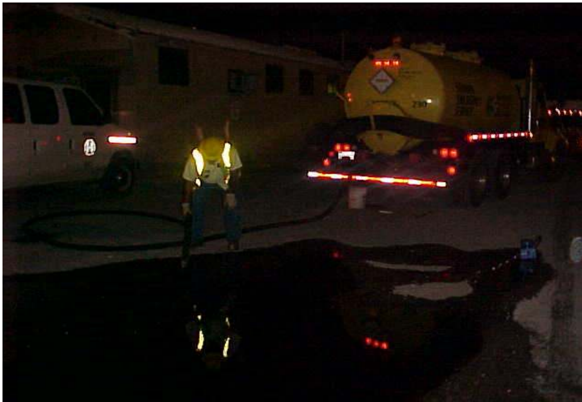
View Northwest - Vacuuming pooled diesel fuel. Radio Shop is displayed in the background.
