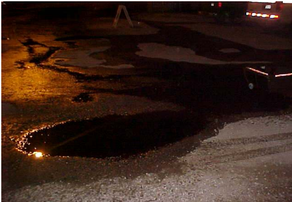
View West - Pooling diesel fuel east of the canopy.
