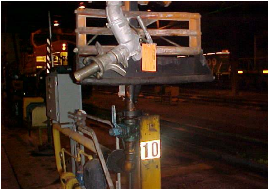
View Southwest - Dispenser 10, tagged out of service.
