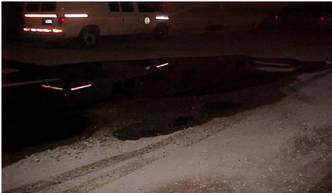
View Northwest - Additional pooling southeast of the Radio Shop.
